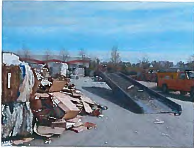
Photo 4. One of the drain inlets onsite Note: the significant amount of material on the asphalt surface
