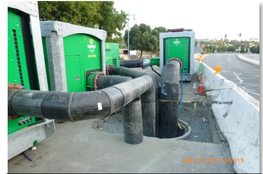
Mare Island Bypass System
