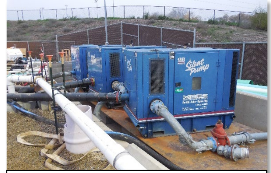
Oak Ave PS Bypass Pumping System
