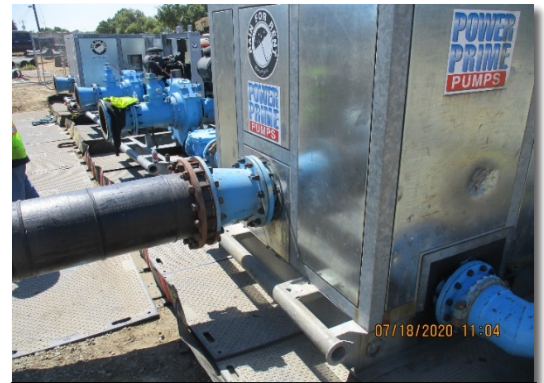
Delta Bypass Pumping System
