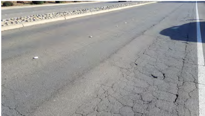
GARDEN HWY, (POOR) – PCI 39
