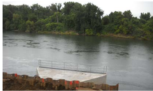
Light Beacons Have Been Secured to the Structure & Warning Signage will also be installed for Boater Safety
